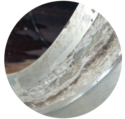
Corrosion caused by use of conventional graphite gaskets
